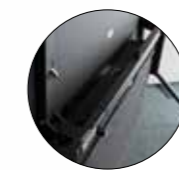
Kabelkanal cable duct
